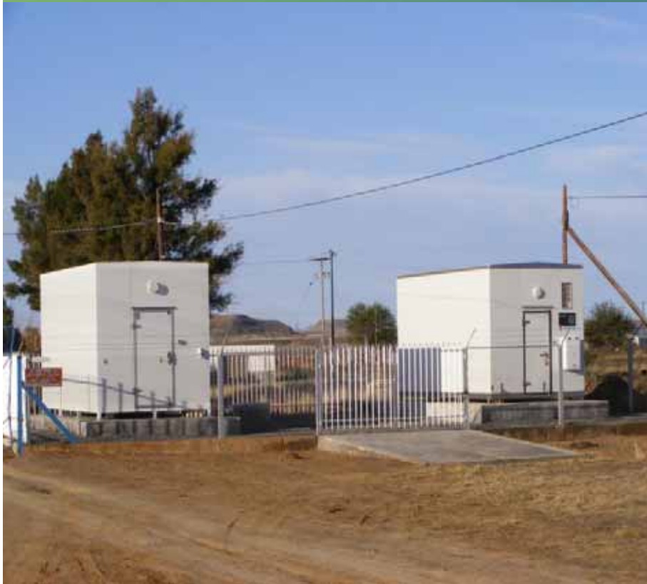
Above: Carnarvon Point of Presence (POP) station (SANReN/SKA interface)
