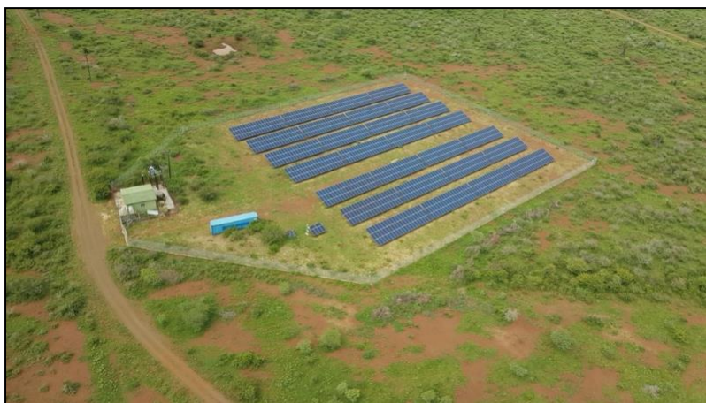
Lower Sabie solar PV plant (Photo: SANParks)
